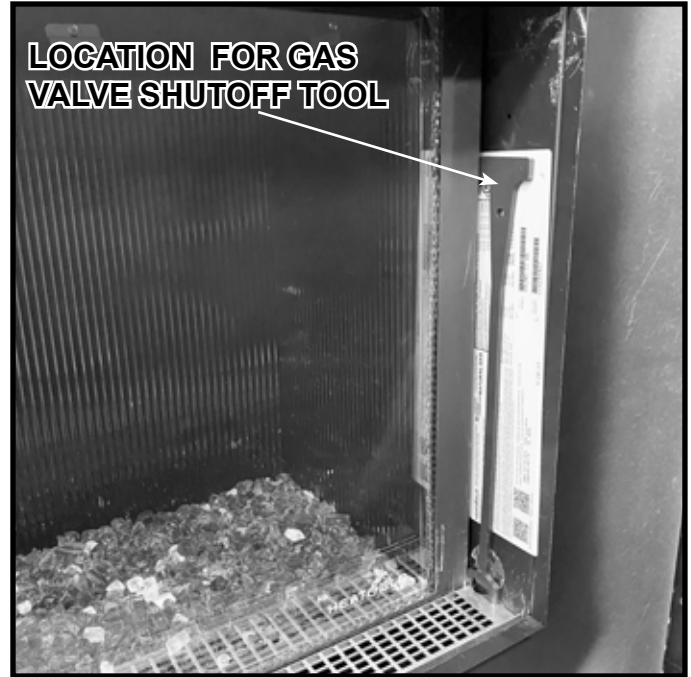
Figure 11.22 Storage Location for Gas Valve Shutoff Tool
