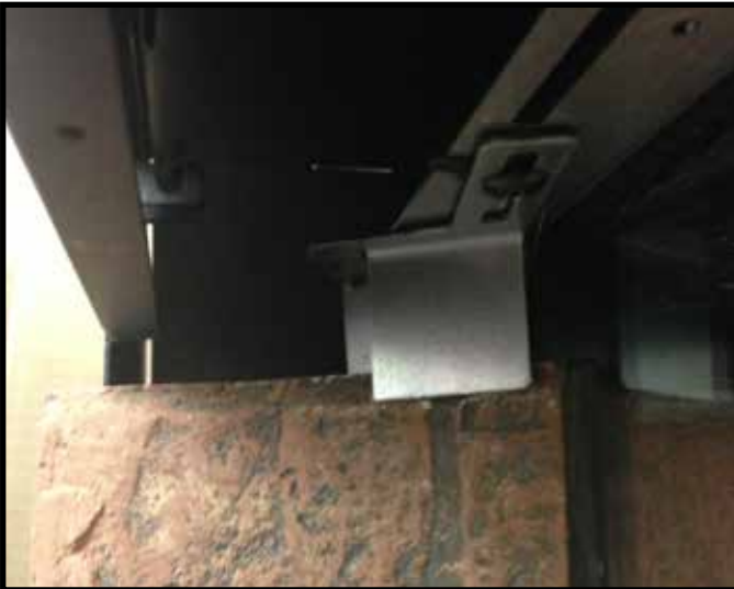
Figure 11.27 Side Refractory Brackets
