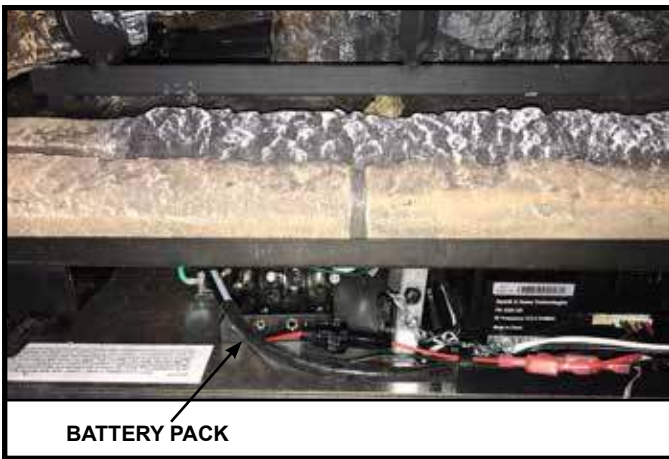
Figure 6.3 Battery Pack Installed
