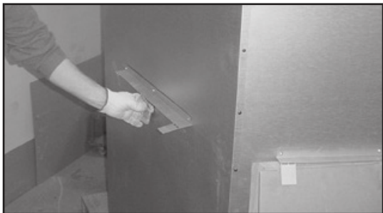
Figure 3.7 Bend Refractory Brackets Back Down
